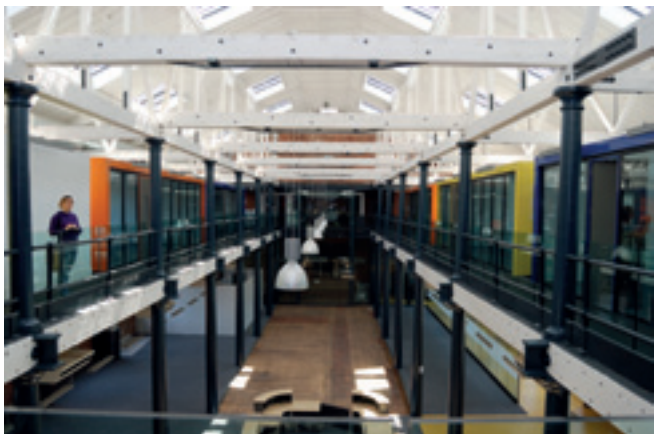
Intumescent paints are often used to enable the retention of structural elements such as these cast iron columns where industrial buildings are converted. The coating must ensure that structural integrity is maintained for long enough to evacuate the building.
